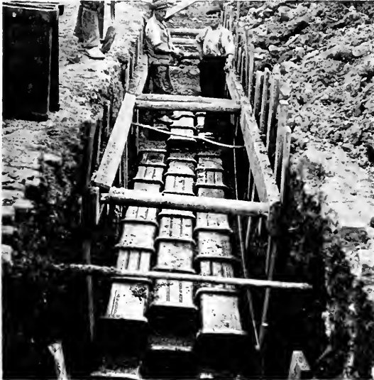
FIG. 8.—CONDUITS AT ENTRANCE TO POWER STATION.
